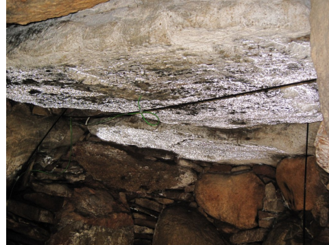
Figure 11: Condensation on the ceiling of the grave chamber caused by unhindered entry of relatively warm and humid ambient air.
